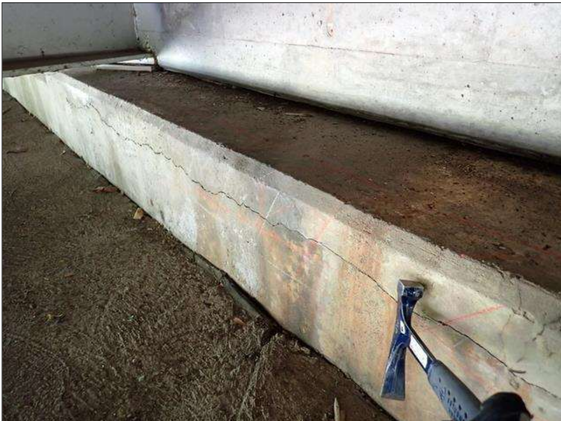
End Bent 2 Cap 1: IN BAY 4, 13 FOOT UP TO 1/8 INCH HORIZONTAL CRACK WITH DELAMINATED AREA 13 FOOT X 9 INCH X 7 INCH ON TOP AND SOUTH FACE.
