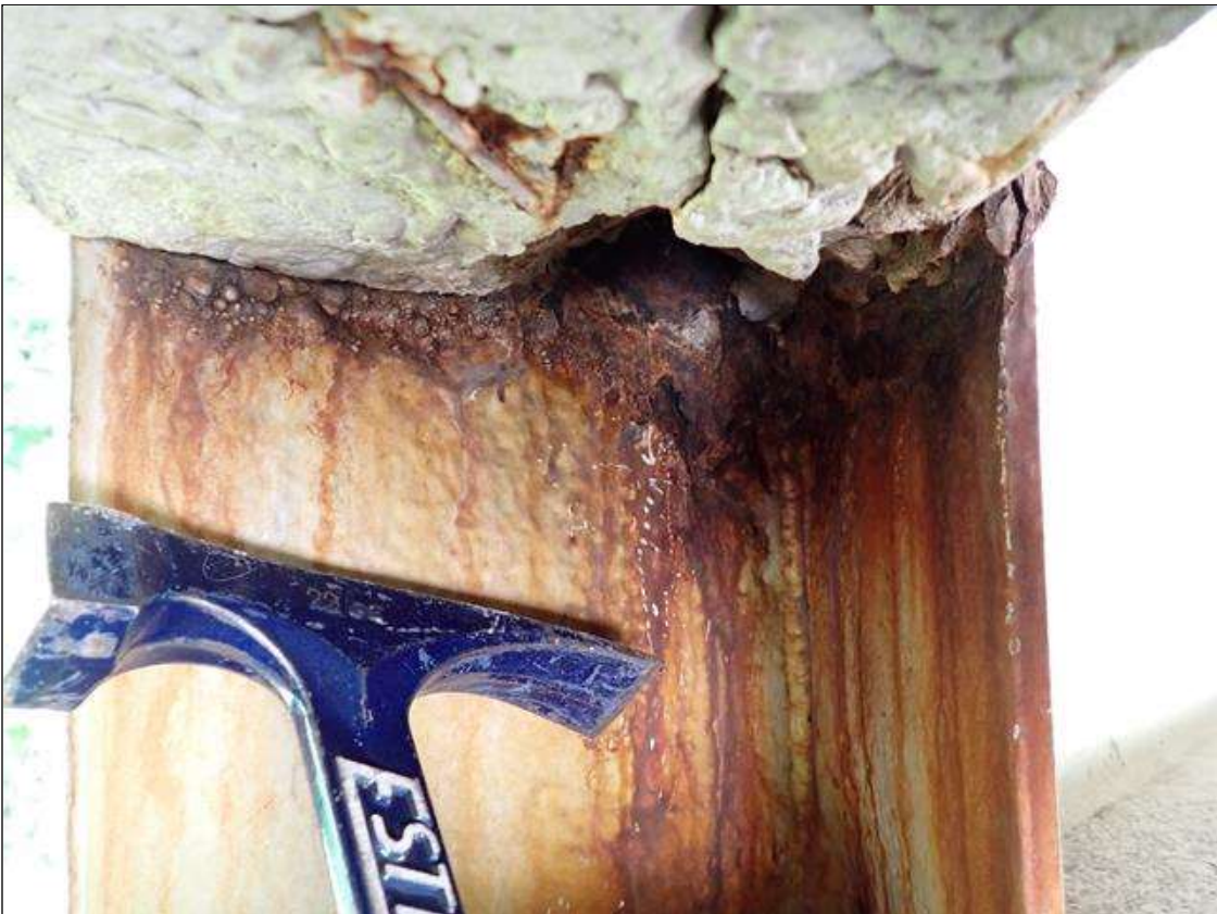
Span 3 Beam 5: at bent 3, corrosion with section loss: web adjacent to diaphragm (9/16 average remaining x 10 inch x 2.5 inch); left stiffener (0.25 inch average remaining x full width x 2.5 inch)
