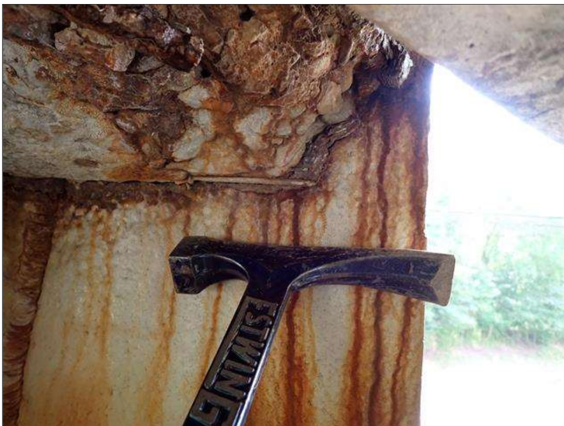
Span 2 Beam 1: at bent 2, pitting with corrosion reactivating: web adjacent to diaphragm (1/16 inch deep x 10 inch x 2 inch)
