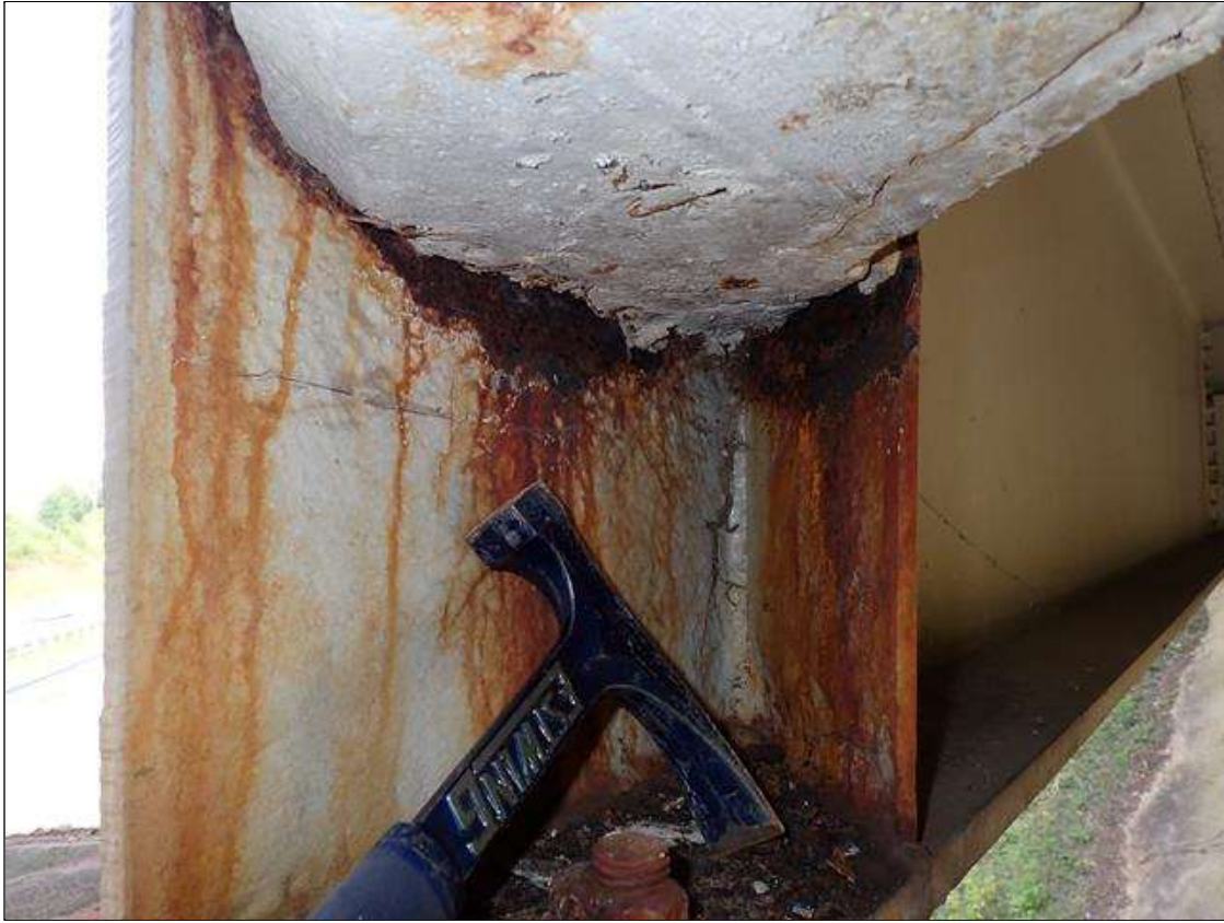
Span 1 Beam 5: at bent 1, corrosion with section loss: web adjacent to diaphragm (9/16 average remaining x 10 inch x 2 inch); left stiffener adjacent to diaphragm (0.25 inch average remaining x full width x 2 inch); left stiffener at base (0.27 inch average remaining x full width x 2 inch); top flange, rust scale (1 foot)
