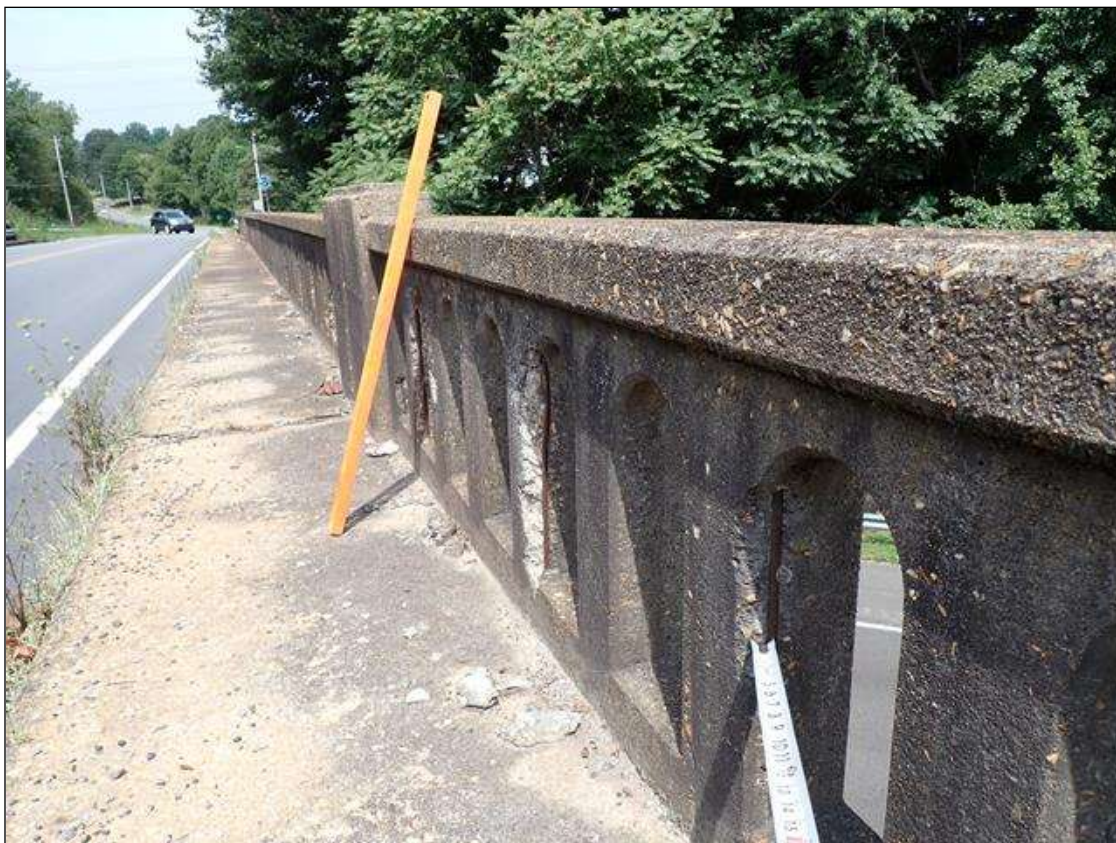
Span 2 Right Bridge Rail: along length of rail, multiple spalls, up to 20 inch x 4 inch x 1 inch deep, some with exposed rusted reinforcing, no loss noted
