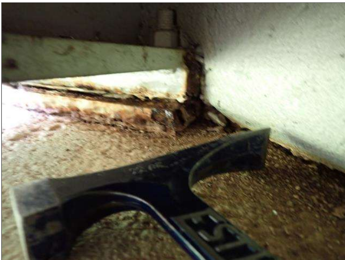
Span 4 Far Bearing 1: surface rust/rust scale
