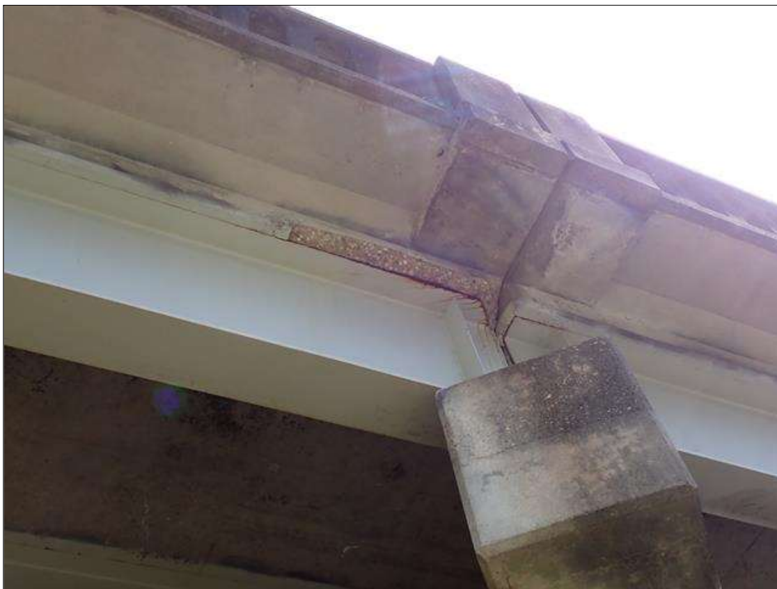
Span 4 Deck: BOTTOM OF DECK WEST SIDE OF BEAM 1 OVER BENT 3 SPALL ALONG TOP FLANGE 7 INCH X 4 FOOT X 1 INCH DEEP.
