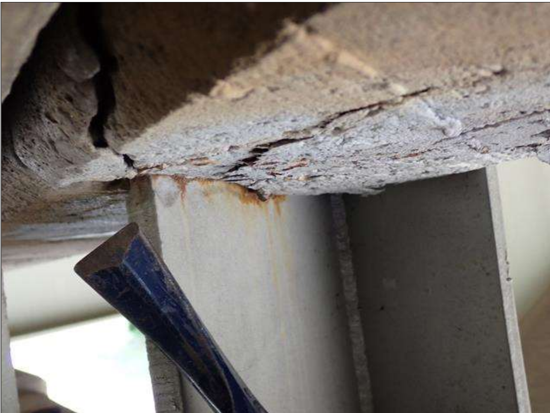
Span 2 Beam 2: at bent 2, corrosion with section loss: web adjacent to diaphragm (5/8 average remaining x 6 inch x 1 inch)
