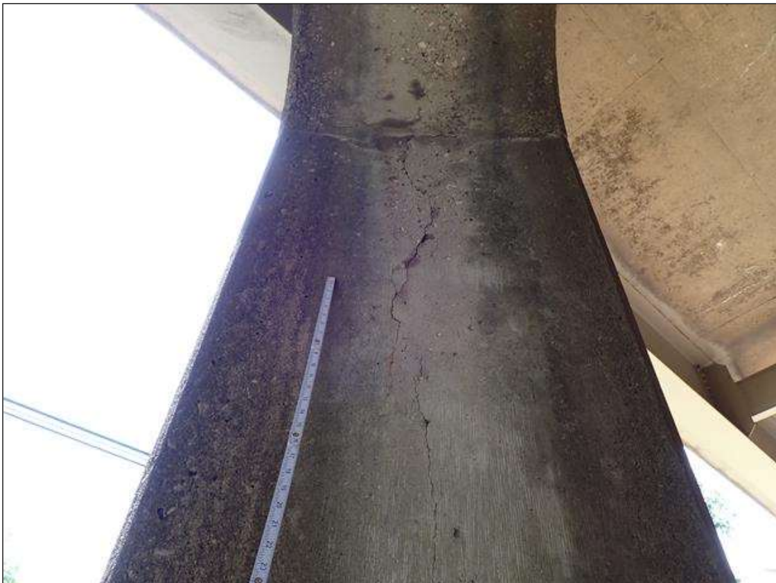
Bent 3 Pile 1: (4) 6 FOOT X UP TO 1/32 INCH VERTICAL CRACKS BEGINNING AT BOTTOM OF CAP AT RANDOM THROUGHOUT.
