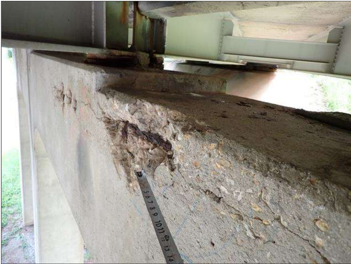
Bent 1 Cap 1: [PAR] 32 INCH X 15 INCH X 3 INCH SPALL WITH EXPOSED PRIMARY REINFORCING [SECTION LOSS UP TO 1/8 INCH] WITH ADJACENT DELAMINATION ON TOP NORTH FACE UNDER BAY 1.
