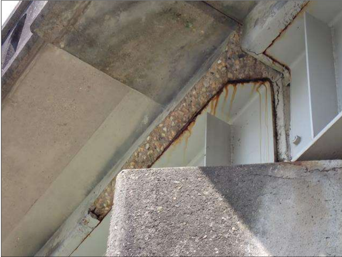
Span 4 Beam 1: (PAR) at bent 3, corrosion with section loss: web adjacent to diaphragm (9/16 inch average remaining x 11 inch x 2 inch); right stiffener (0.15 inch average remaining x full width x 3 inch) with corrosion holes (up to 1/4 inch diameter); west face top flange, rust scale
