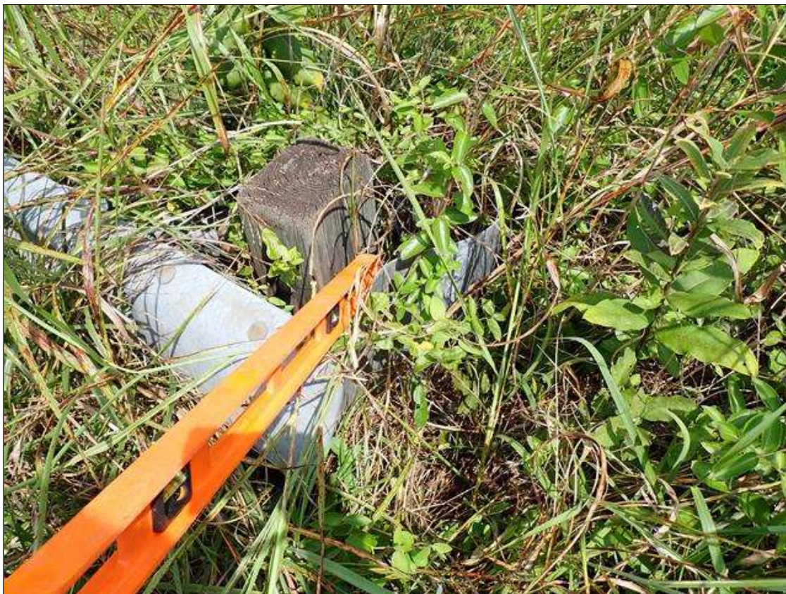
(PAR) southeast guardrail termination, impact damage
