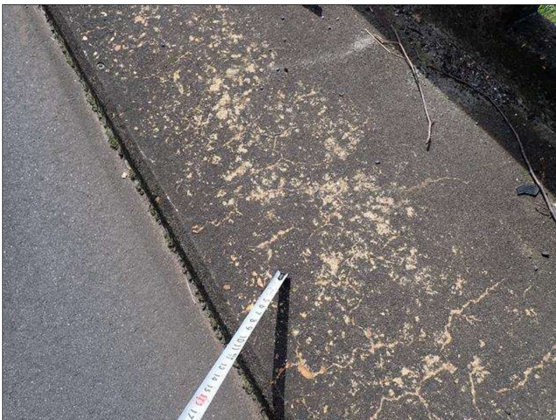
Span 4 Left Bridge Rail: along the length of sidewalk, transverse cracks (hairline x full width) and map cracks (hairline) at random
