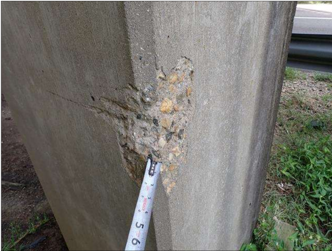
Bent 2 Pile 3: BENT 2 SOUTHEAST CORNER OF COL 3 HAS SPALL AREA 38 INCH ABOVE THE GROUND LINE AND 5 INCH X 5 INCH X 12 INCH X 1 INCH DEEP
