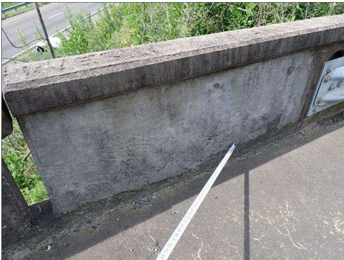
Span 4 Left Bridge Rail: PATCHED AREA 9 FOOT FROM END BENT 2 OVER A 6 FOOT LONG AREA.
