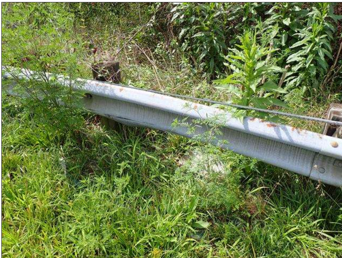
(PAR) northwest guardrail 25 foot from end bent 1, impact damage (6 foot)
