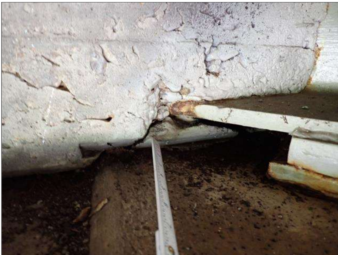
End Bent 2 Abutment: along the length of the abutment, at bottom flange penetrations, spalls/delaminations (8 inch x 4 inch x 1.5 inch deep)
