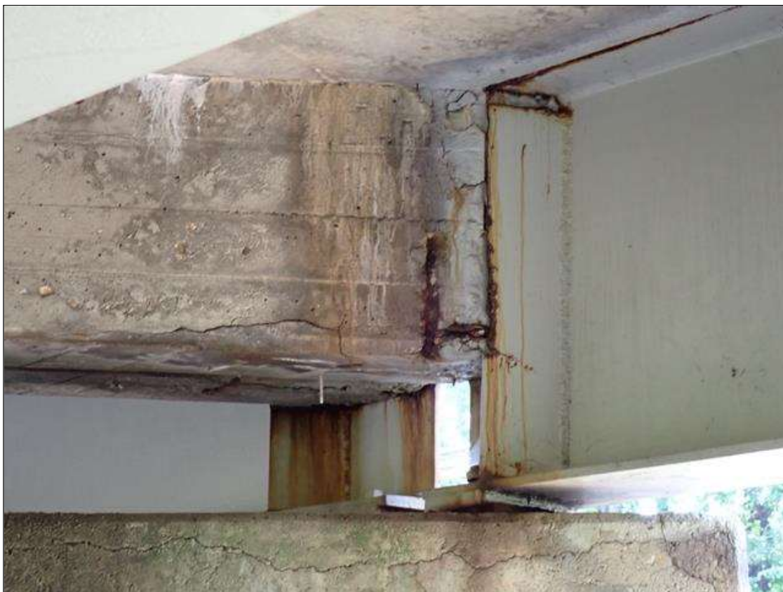
Span 4 Beam 1: 8 INCH X 1 FOOT X 1 INCH SPALL WITH EXPOSED REINFORCING WITH ADJACENT CRACKS UP TO 1/8 INCH BAY 1 IN BENT 3 DIAPHRAGM.
