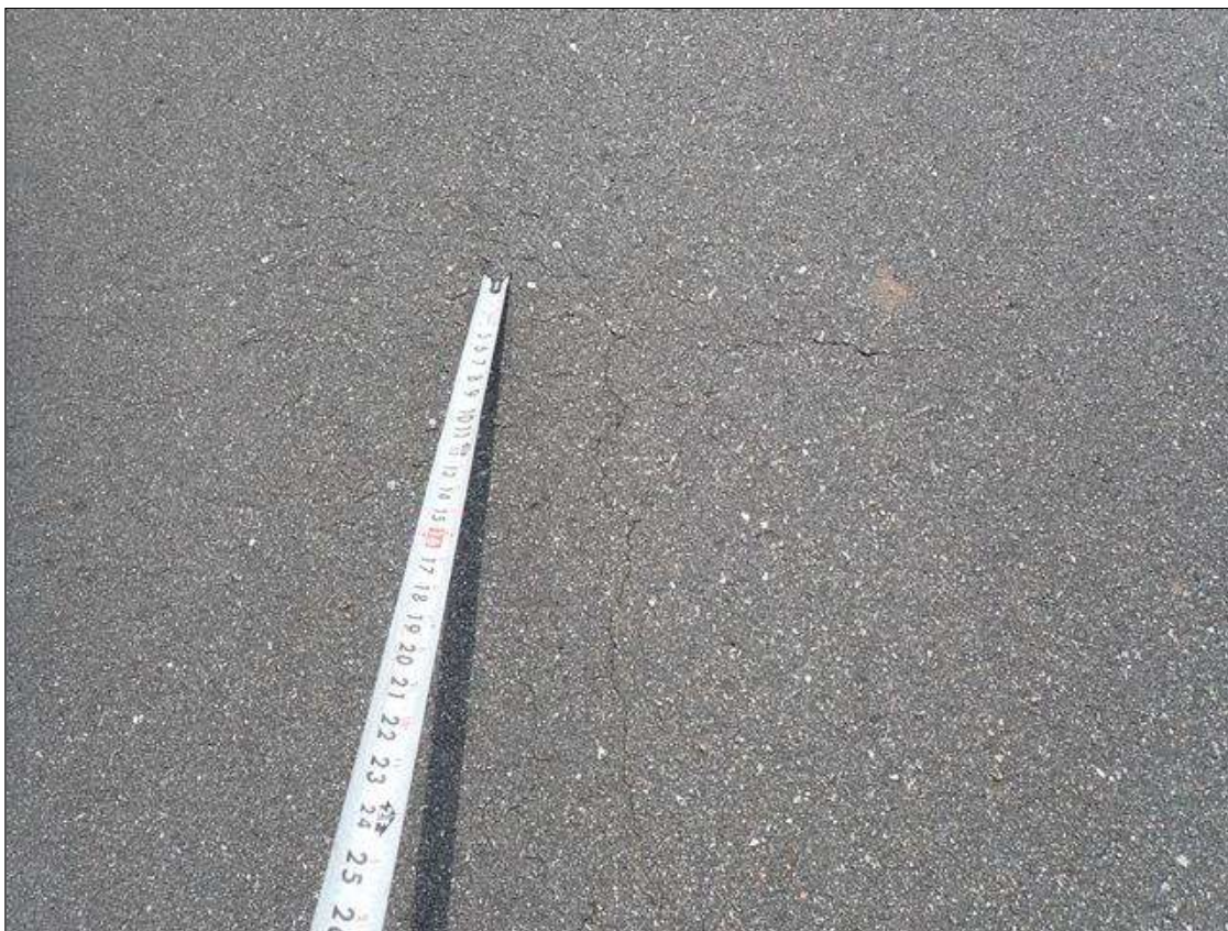
Span 2 Wearing Surface: throughout asphalt wearing surface, transverse and longitudinal cracks (up to 1/32 inch x 5 foot) at random
