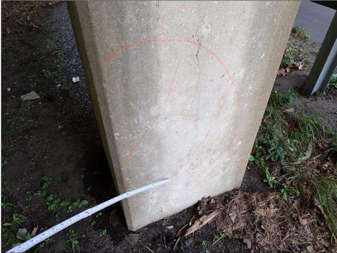
Bent 3 Pile 2: 36 INCH X 24 INCH CRACKED DELAMINATION AREA WITH CRACKS UP TO 1/32 INCH ON WEST FACE NEAR GROUND LINE.
