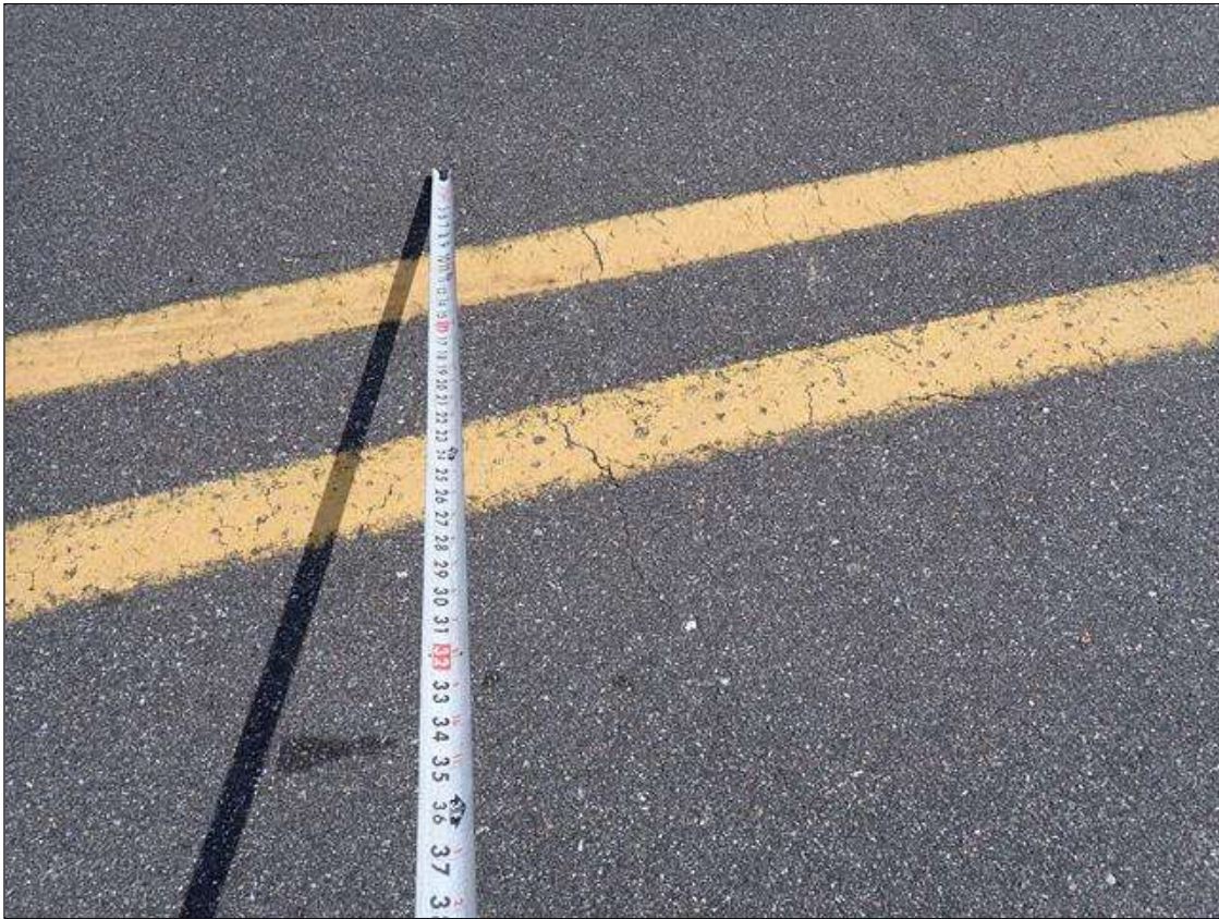
Span 4 Wearing Surface: throughout asphalt wearing surface, transverse and longitudinal cracks (up to 1/32 inch x 5 foot) at random
