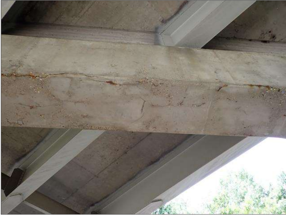
Bent 2 Cap 1: (PAR) 3 FOOT X UP TO 1/8 INCH LONGITUDINAL CRACK WITH RUST STAINING WITH ADJACENT DELAMINATIONS UP TO 5 FOOT X FULL WIDTH SOUTH AND BOTTOM FACES UNDER BAY 3
