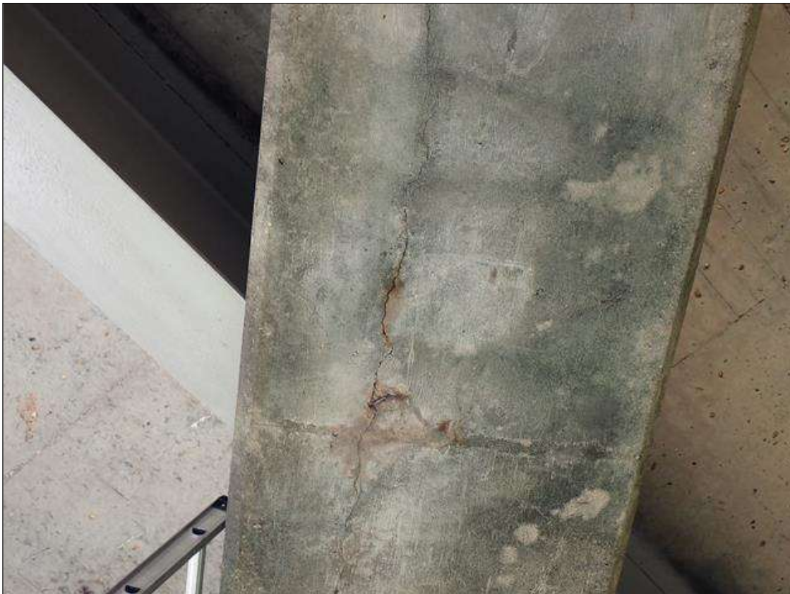
Bent 3 Cap 1: (PAR) UNDERSIDE OF CAP, 10 FOOT UP TO 1/16 INCH LONGITUDINAL CRACK WITH RUST STAINING UNDER BEAM 2, SIMILAR UNDER BEAM 4.
