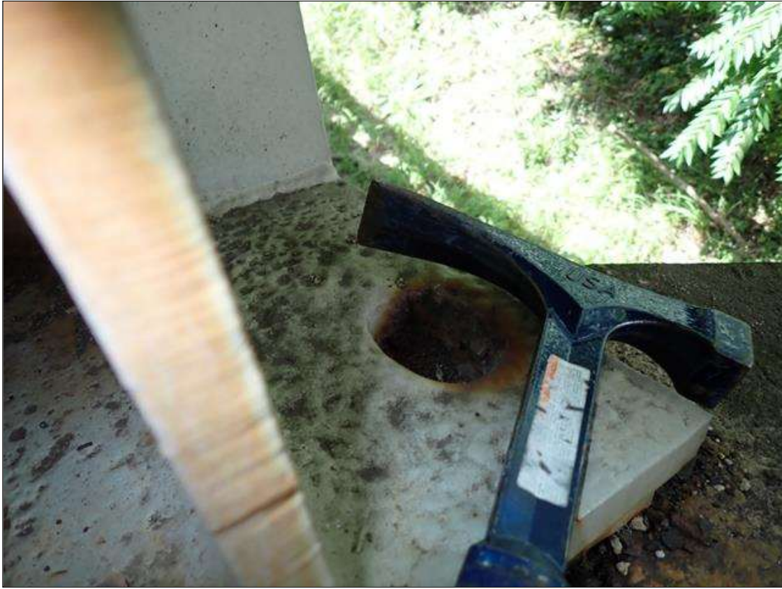
Span 4 Near Bearing 5: (PAR) right anchor rod, sheared/missing
