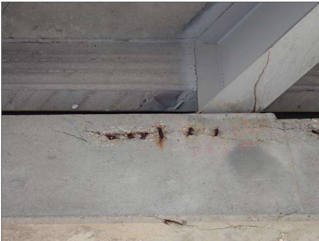
Bent 1 Cap 1: (PAR) 10 INCH X 48 INCH X 2 INCH DEEP SPALL/DELAMINATION WITH EXPOSED RUSTED REBAR NEAR TOP OF CAP, NORTH FACE BELOW BEAM 2
