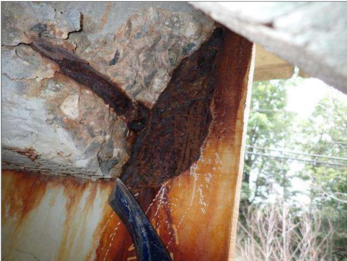
Span 1 Beam 1: at bent 1, corrosion with section loss: web adjacent to diaphragm (9/16 average remaining x 3.5 inch x 8 inch)
