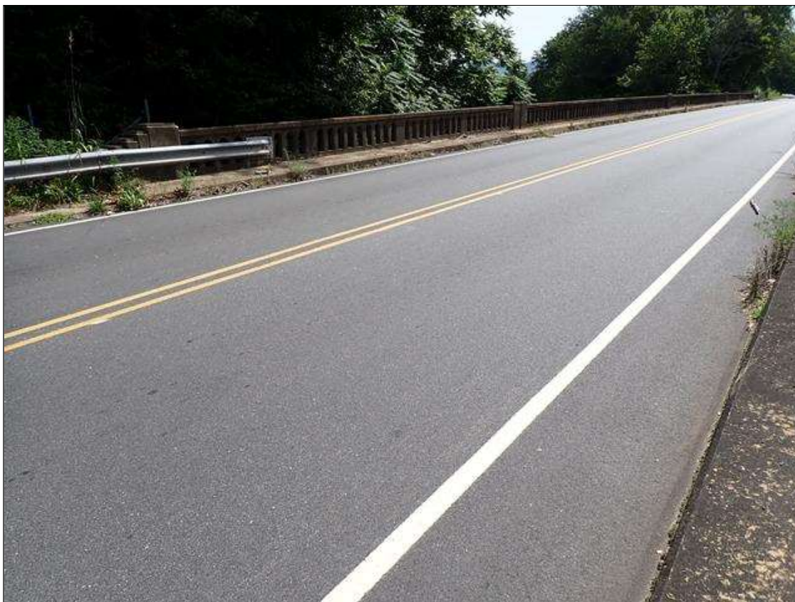
Span 4 Wearing Surface: PREVIOUSLY REPAIRED SEALED MAP & TRANSVERSE CRACKS AT RANDOM THROUGHOUT.
