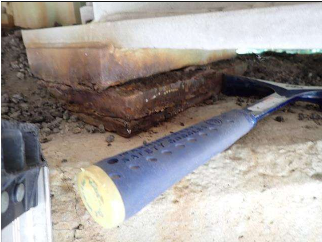
Span 3 Beam 3 - Far Bearing 3: rust scale
