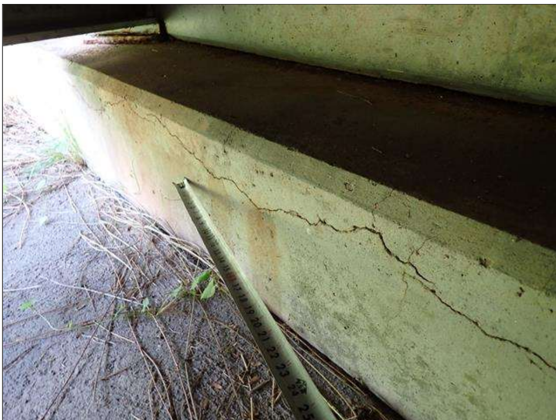
End Bent 2 Cap 1: 5 FOOT X UP TO 1/8 INCH HORIZONTAL CRACK UNDER BEAM 1
