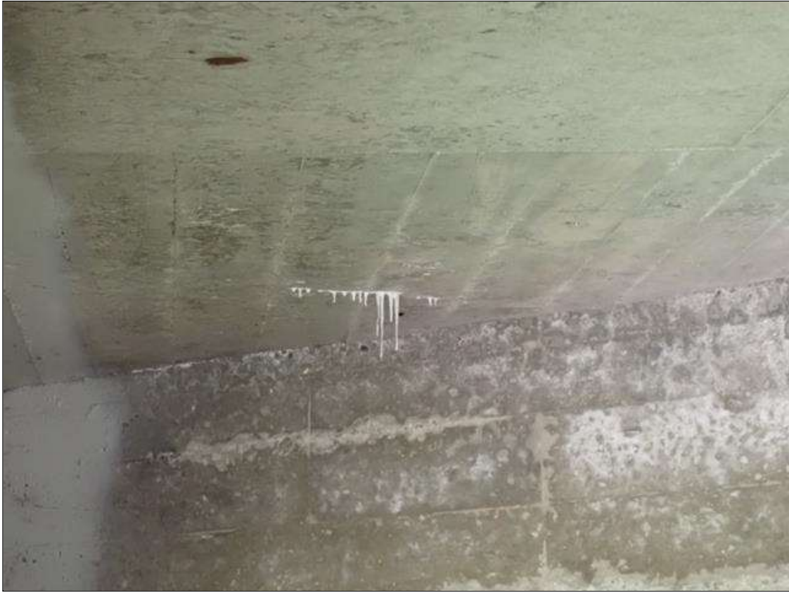
Span 1 Deck: (PAR) EFFLORESCENCE WITH SOME BUILDUP AT RANDOM THROUGHOUT UNDERSIDE OF DECK.
