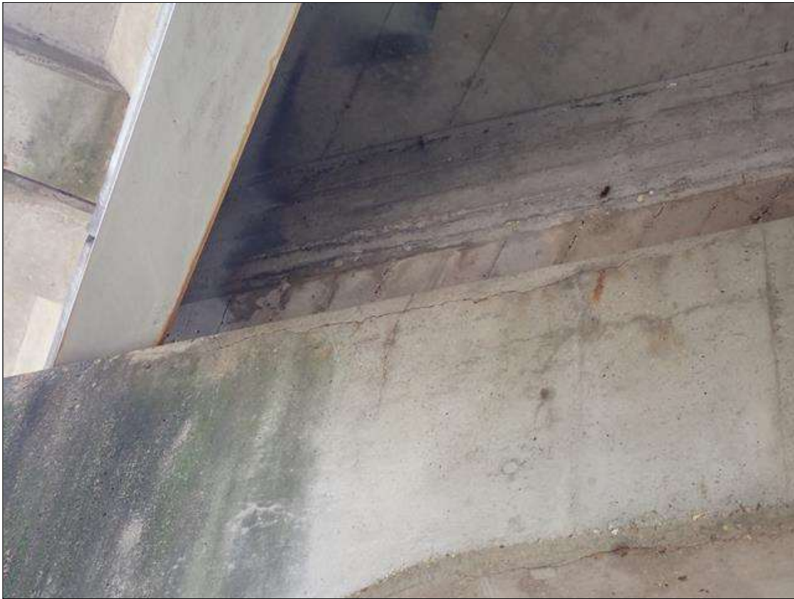
Bent 2 Cap 1: (PAR) BENT 2 NORTH FACE OF CAP HAS A HORIZONTAL CRACK [UP TO 1/8 INCH] WITH RUST STAIN WITH ADJACENT DELAMINATED AREA ALONG TOP EDGE OF CAP BETWEEN BEAM 4 AND BEAM 5 5 INCH TO 20 INCH DOWN FACE 88 INCH LONG AND 4 INCH ON TOP.
