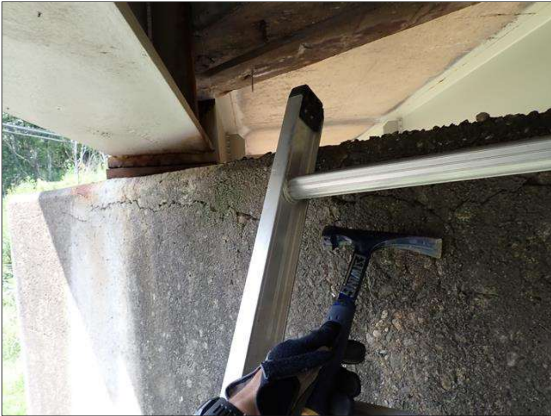
Bent 3 Cap 1: SOUTH AND NORTH FACE (2) UP TO 8 FOOT X 1/16 INCH HORIZONTAL CRACK UNDER BAY 1, SIMILAR BAY 4.
