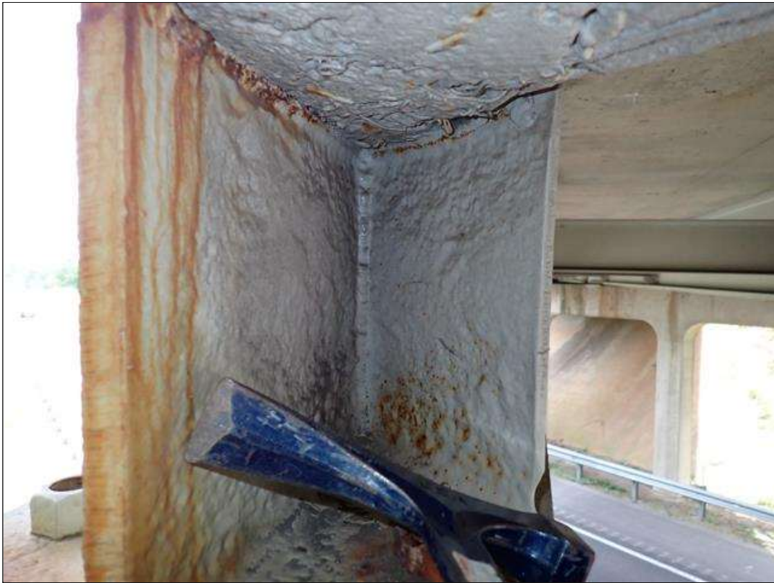
Span 2 Beam 5: at bent 2, corrosion with section loss: web (5/8 average remaining x 10 inch x full height); left stiffener (0.30 inch average remaining x full width x full height)
