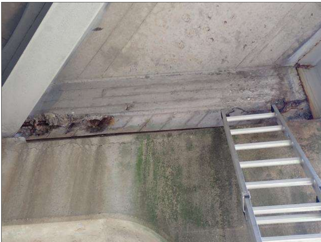
Span 3 Beam 1: at bent 2, bay 1 end diaphragm, (2) spall/delamination (up to 3 foot x 10 inch x 2 inch deep) with exposed rusted rebar
