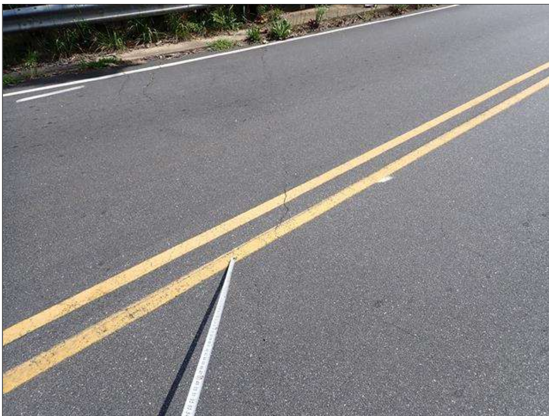
Span 4 Wearing Surface: at end bent 2, transverse cracks (up to 1/32 inch x 15 foot)
