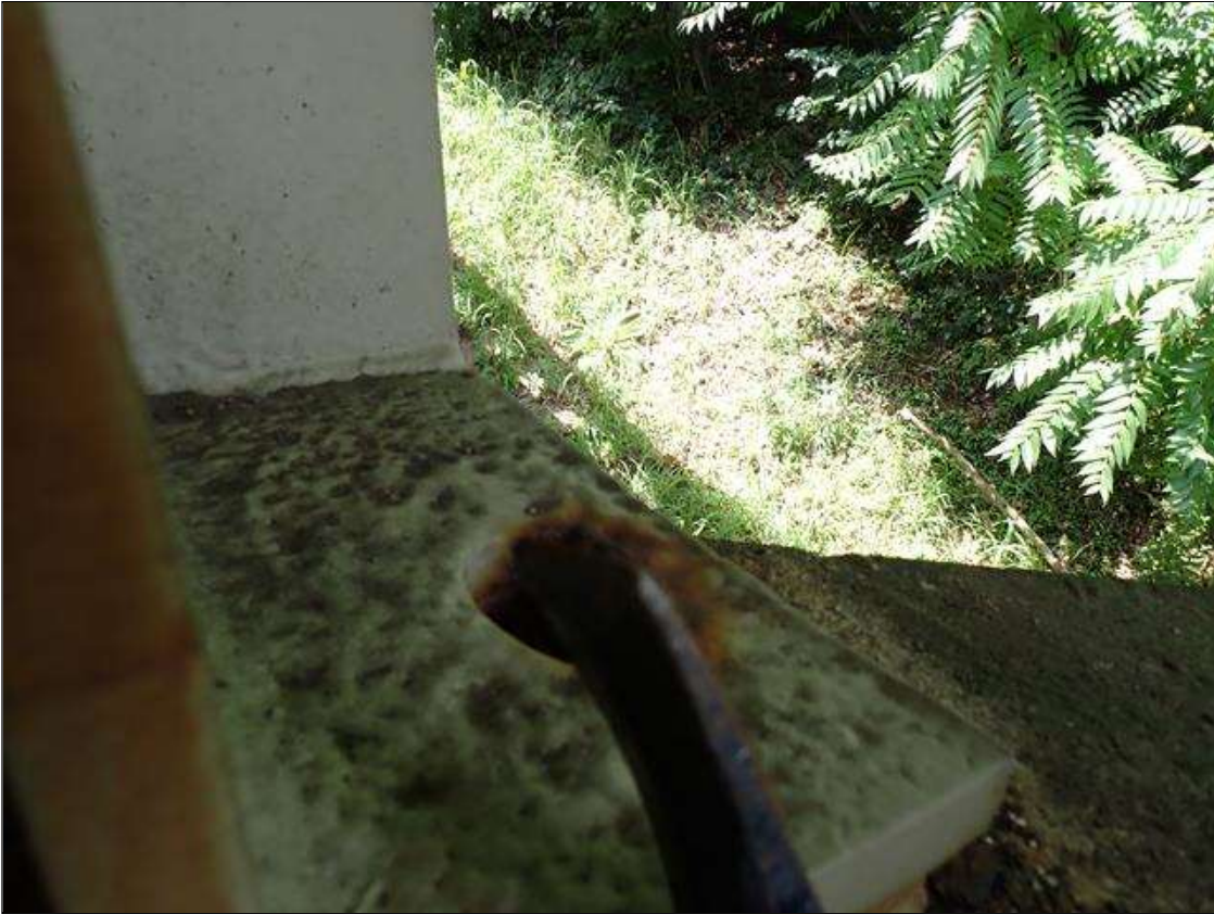
Span 4 Beam 5: at bent 3, pitting with corrosion reactivating: web adjacent to diaphragm (up to 1/16 inch deep x 10 inch x 2.5 inch); bottom flange (1/8 inch deep x 1 foot)
