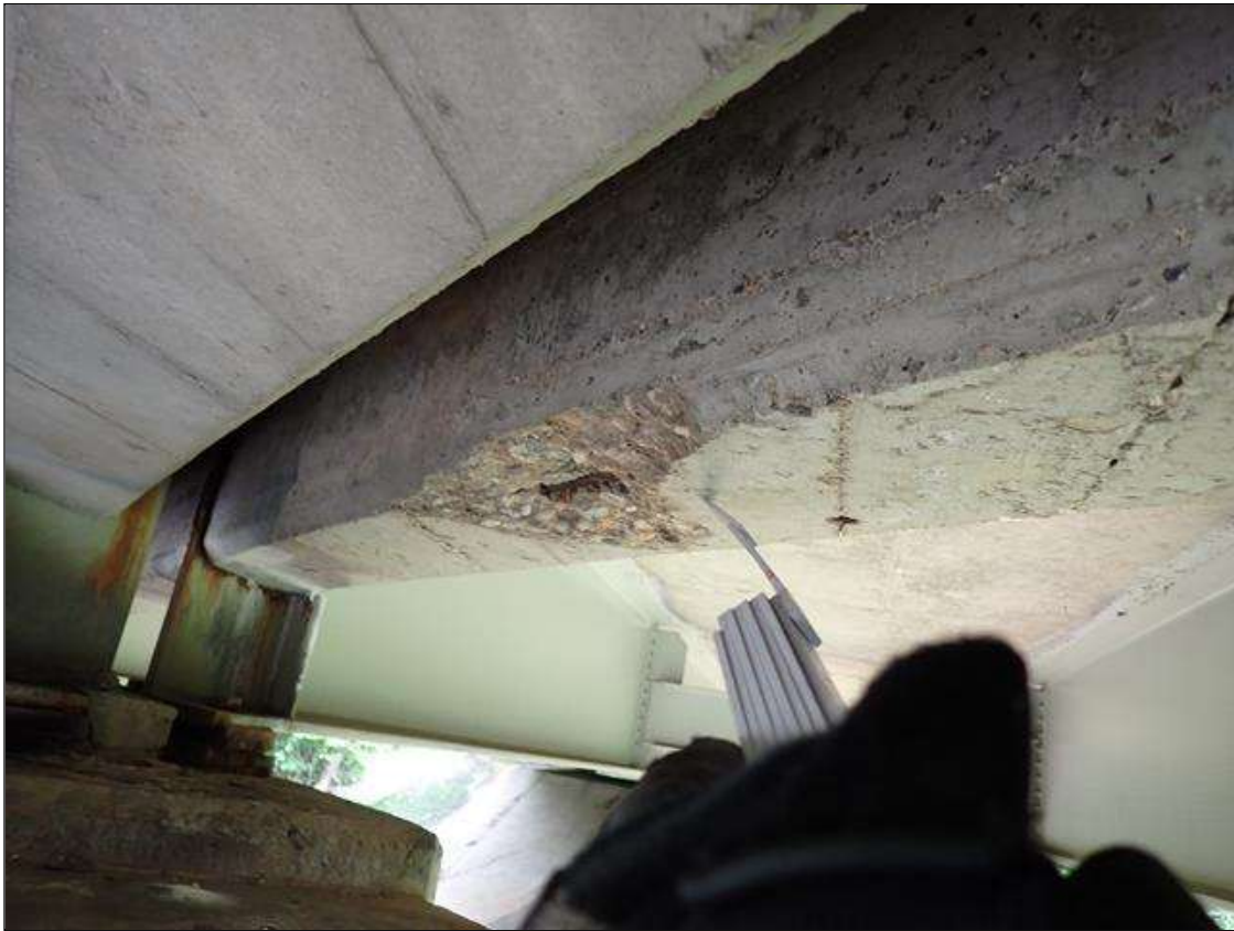
Span 1 Beam 1: at bent 1, bay 1 diaphragm, (2) spall/delamination (up to 2 foot x 8 inch x 2.5 inch deep) with exposed rusted rebar
