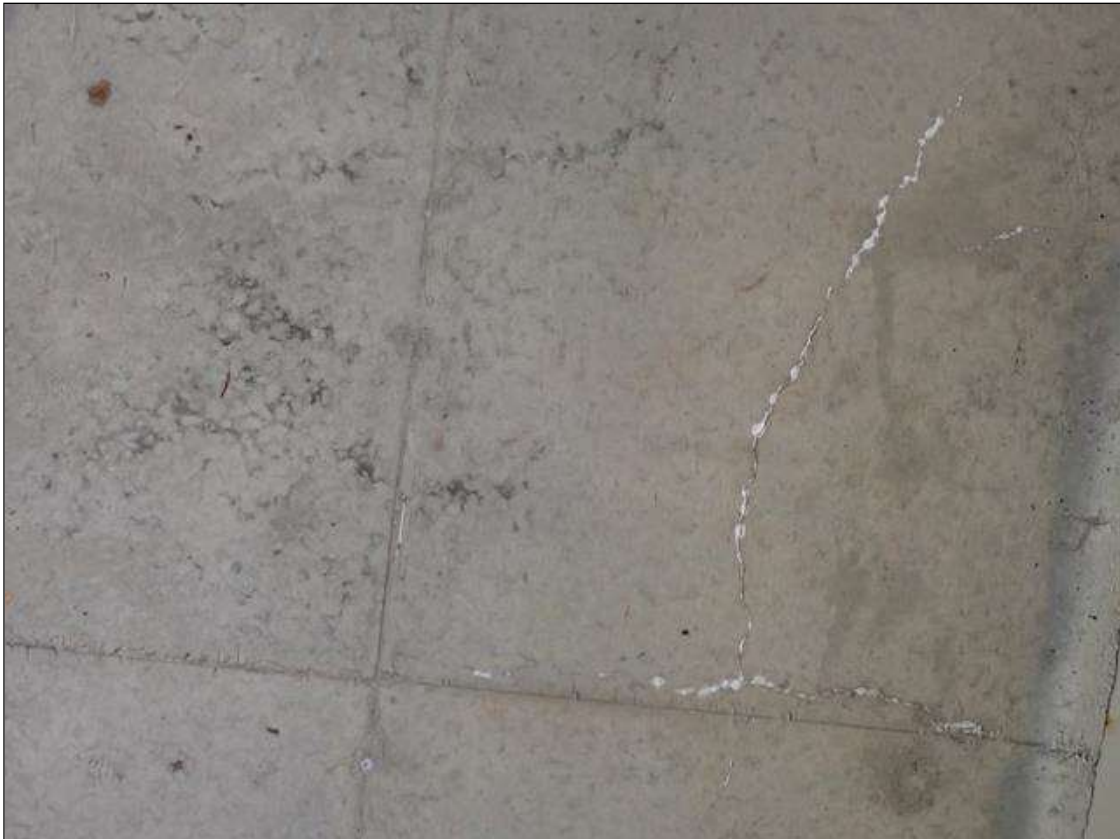
Span 3 Deck: SPAN 3 BOTTOM OF DECK HAS SCATTERED AREAS IN ALL BAYS OF MAP CRACKING WITH EFFLORESCENCE
