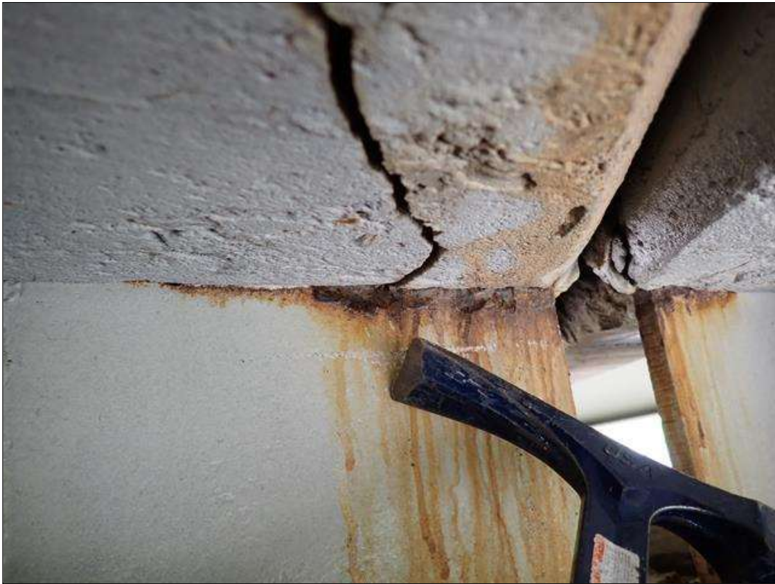
Span 3 Beam 3: at bent 2, web adjacent to diaphragm, rust scale (8 inch)
