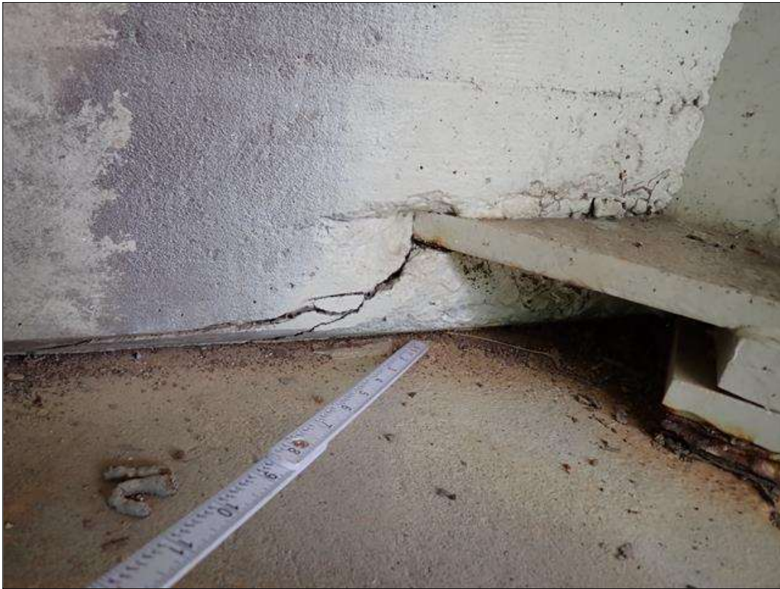
End Bent 1 Abutment: along the length of the abutment, at bottom flange penetrations, spalls/delaminations (12 inch x 5 inch x 1 inch deep)
