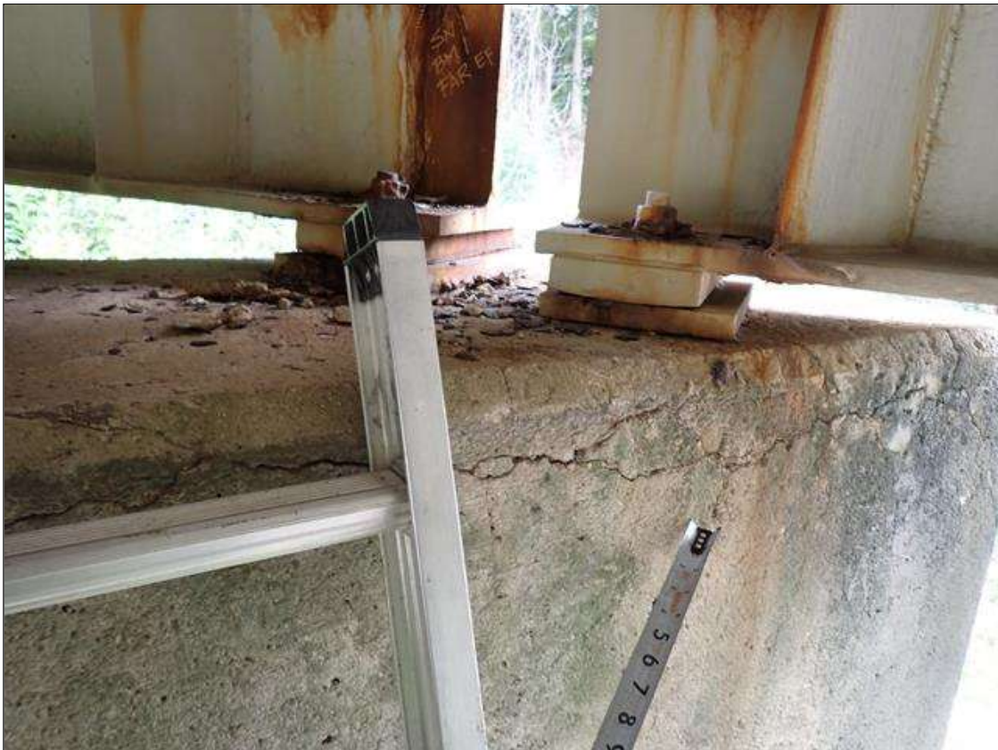
Bent 1 Cap 1: UP TO 14 FOOT X 1/8 INCH HORIZONTAL CRACKS AT RANDOM THROUGHOUT ON SOUTH FACE AND UNDERSIDE
