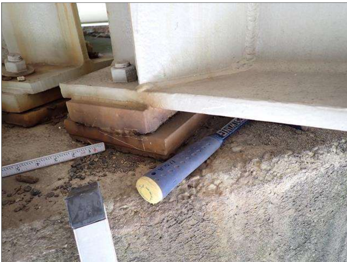
Span 3 Beam 2 - Far Bearing 2: surface rust
