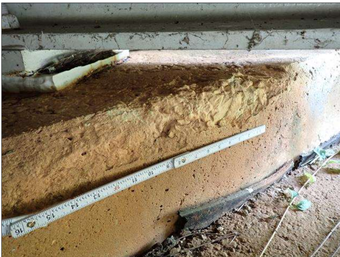
End Bent 1 Cap 1: below beam 1, spall (1 foot x 3 inch x 1/2 inch deep)
