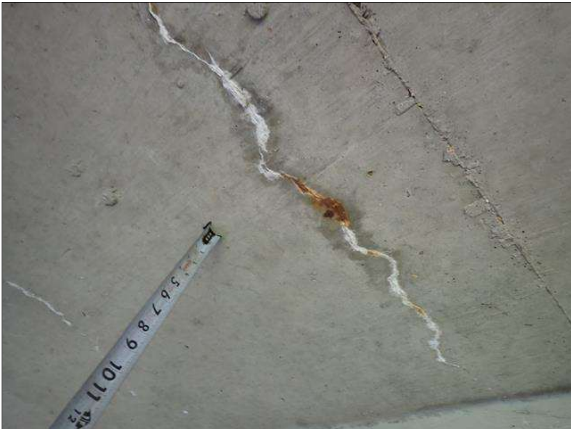
Span 4 Deck: (PAR) in bay 1 near end bent 2, transverse crack (hairline x full bay width) with efflorescence and rust stains; in bay 4 near midspan, transverse cracks (hairline x full bay width) with efflorescence buildup
