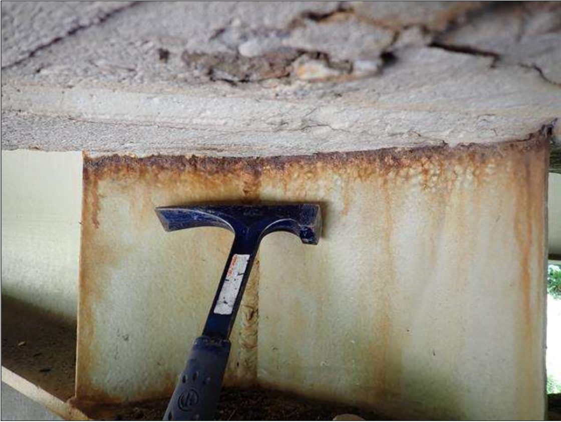
Span 4 Beam 3: at bent 3, pitting with corrosion reactivating: web adjacent to diaphragm (1/16 inch deep x 10 inch x 2 inch); left stiffener (1/16 inch deep x full width x 2 inch)
