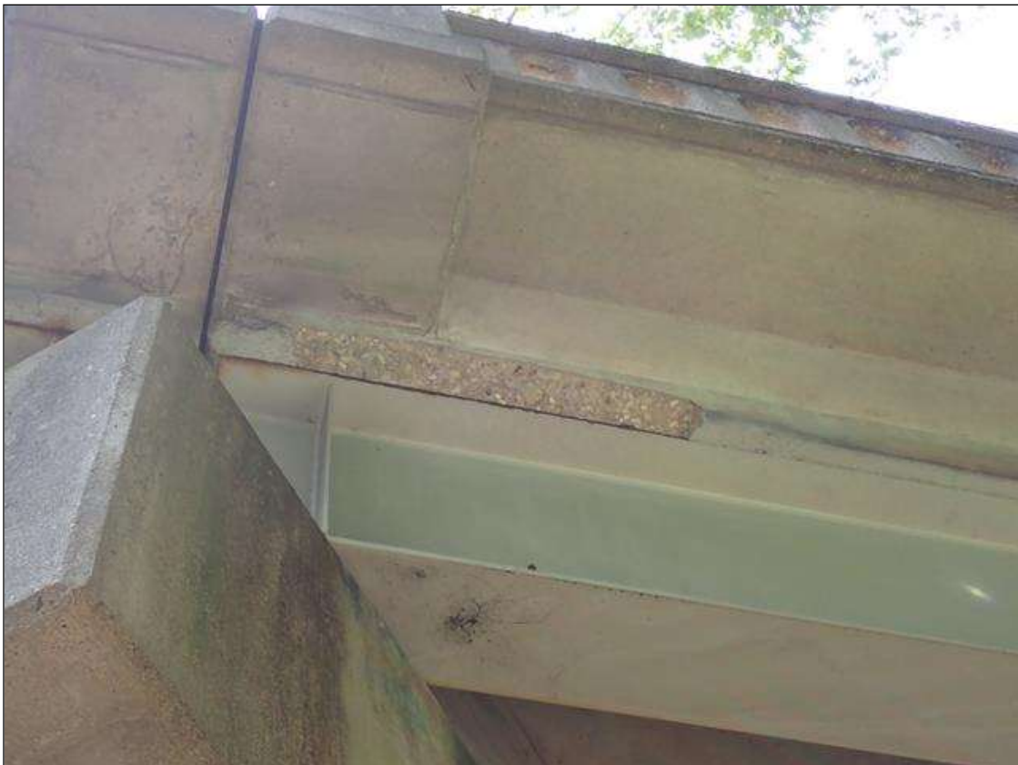
Span 4 Deck: BOTTOM OF DECK EAST SIDE OF BEAM 5 OVER BENT 3 SPALL ALONG TOP FLANGE 7 INCH X 4 FOOT X 1 INCH DEEP.
