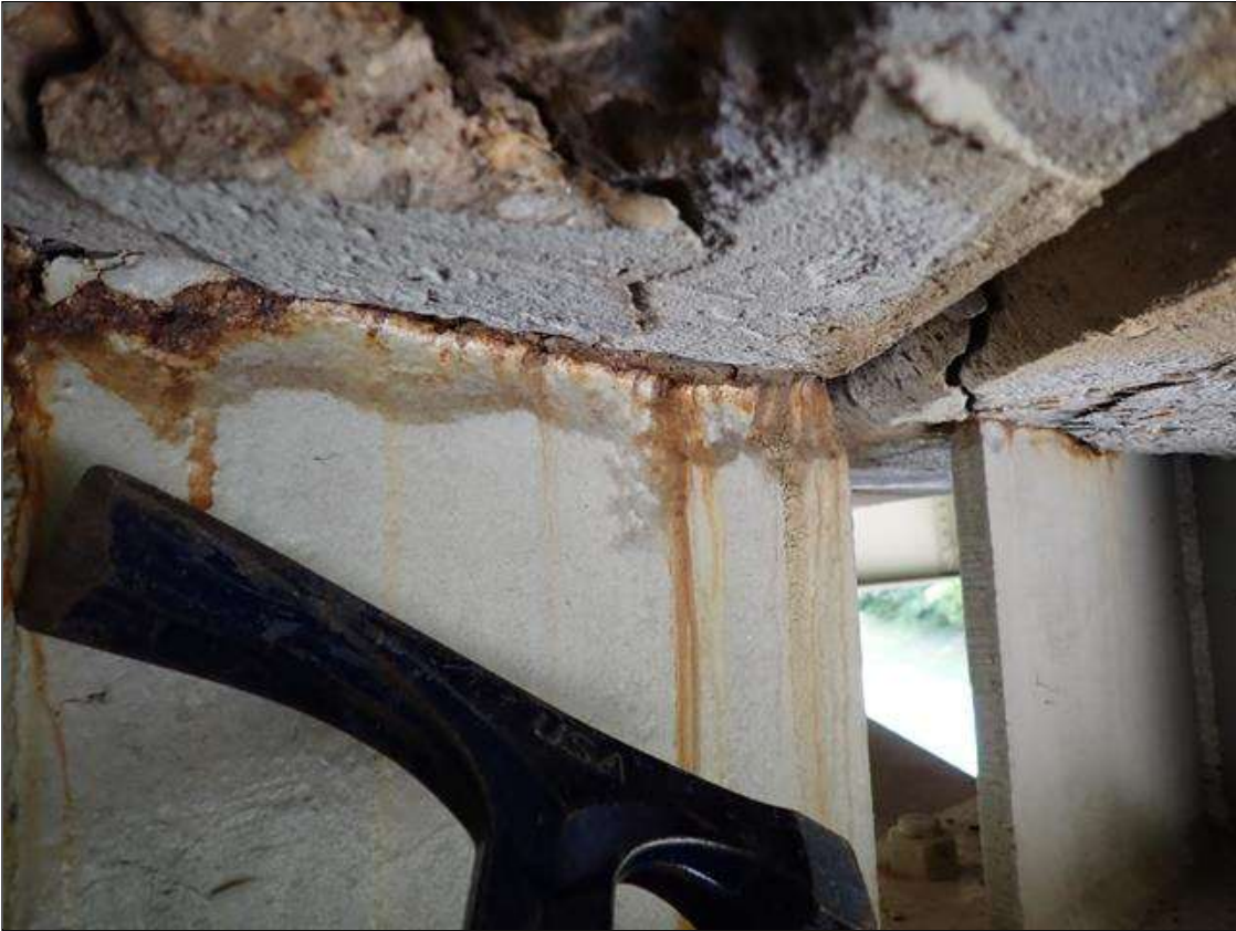
Span 3 Beam 2: (PAR) at bent 2, corrosion with section loss: web adjacent to diaphragm (1/2 average remaining x 10 inch x 1.5 inch)
