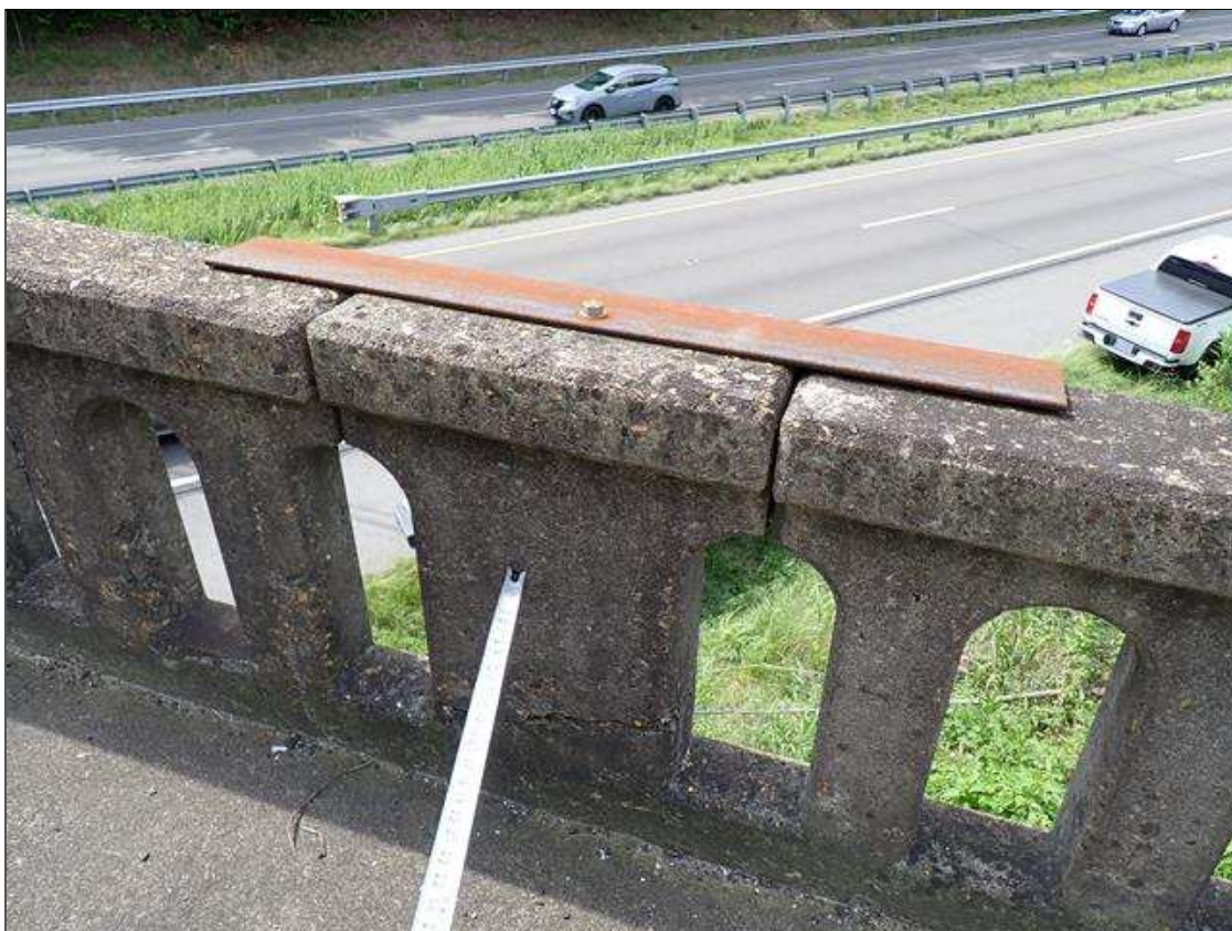
Span 4 Left Bridge Rail: previously repaired crack on post at 24 foot from bent 3
