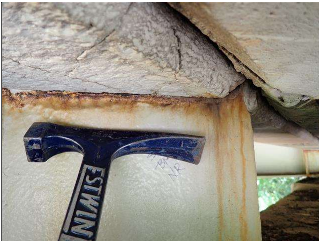
Span 4 Beam 2: at bent 3, corrosion with section loss: web adjacent to diaphragm (9/16 average remaining x 10 inch x 2 inch)
