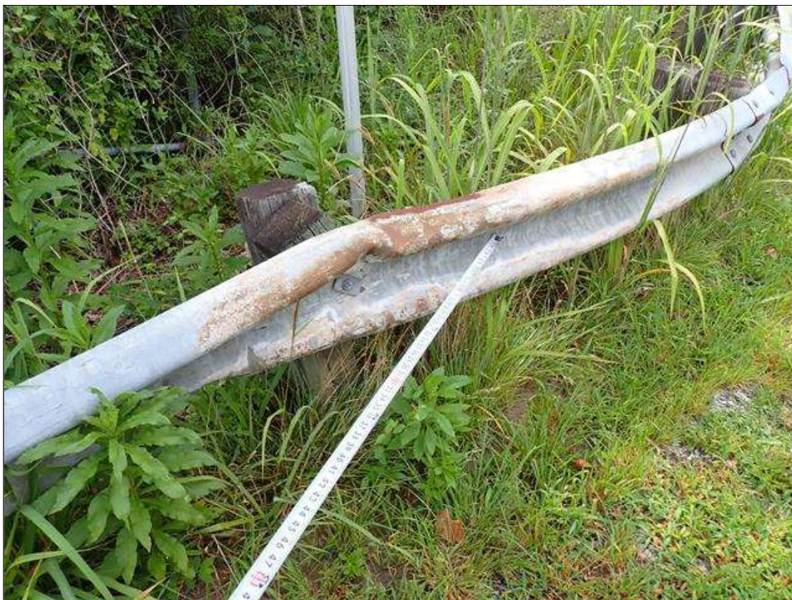
(PAR) northeast guardrail 25 foot from termination, impact damage (4 foot)
