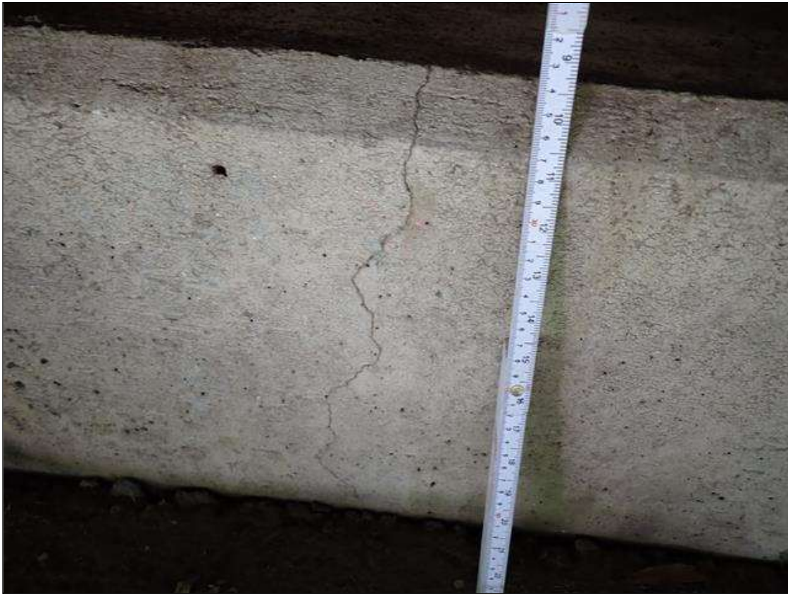
End Bent 2 Cap 1: along length of cap, multiple vertical cracks, up to full height x 1/32 inch
