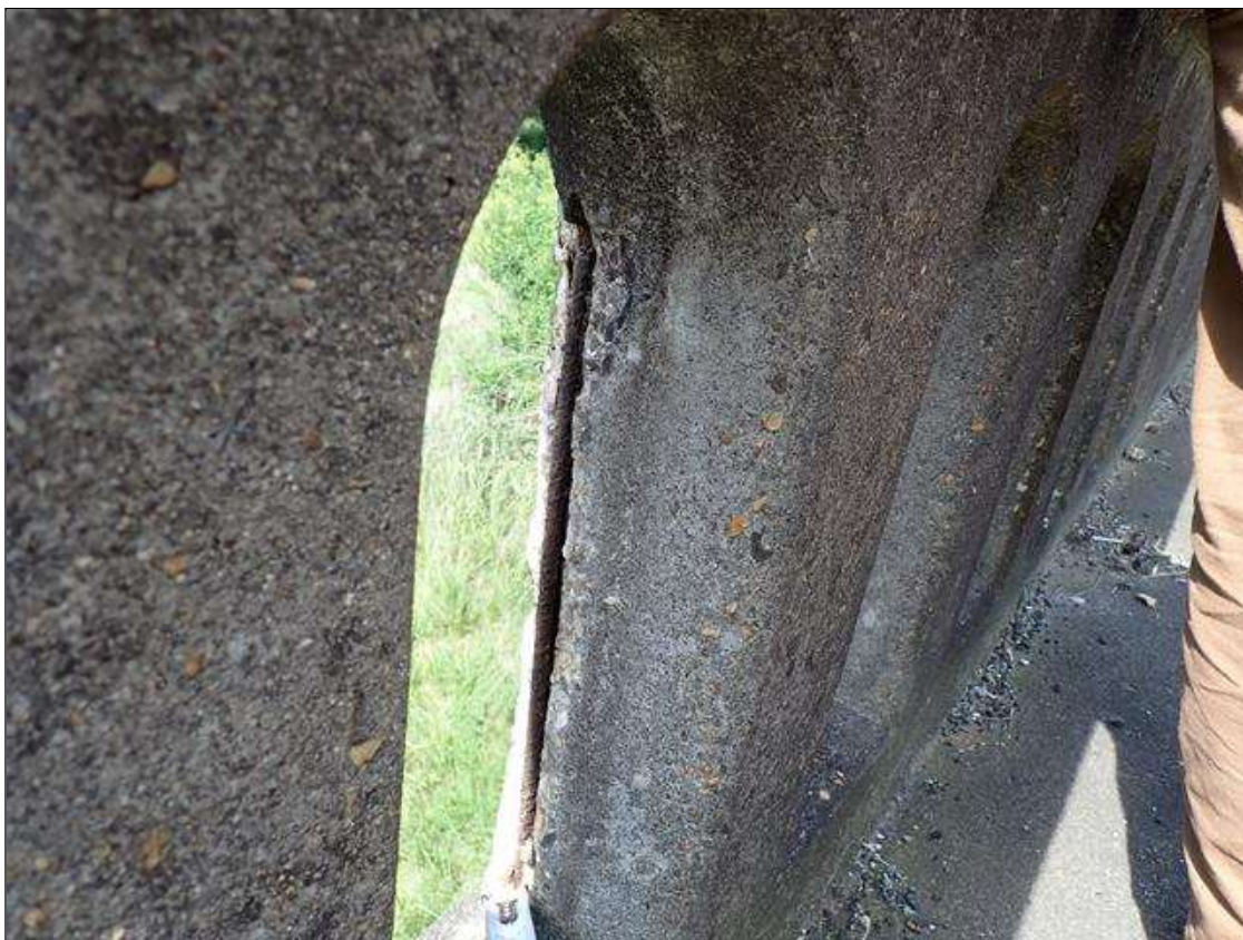
Span 4 Left Bridge Rail: along length of rail, multiple spalls, up to 20 inch x 3 inch x 1 inch deep, some with exposed rusted reinforcing, no loss noted
