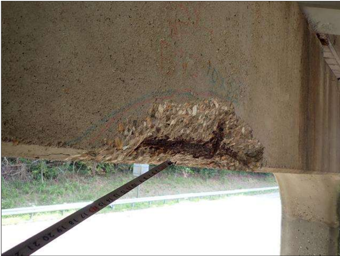
Bent 2 Cap 1: (PAR) 3 FOOT X UP TO 7 INCH X 8 INCH X 3 INCH DEEP SPALL WITH EXPOSED REINFORCING WITH APPROXIMATELY 25 PERCENT LOSS AND ADJACENT DELAMINATION UNDER BAY 2 NORTH AND BOTTOM FACES.
