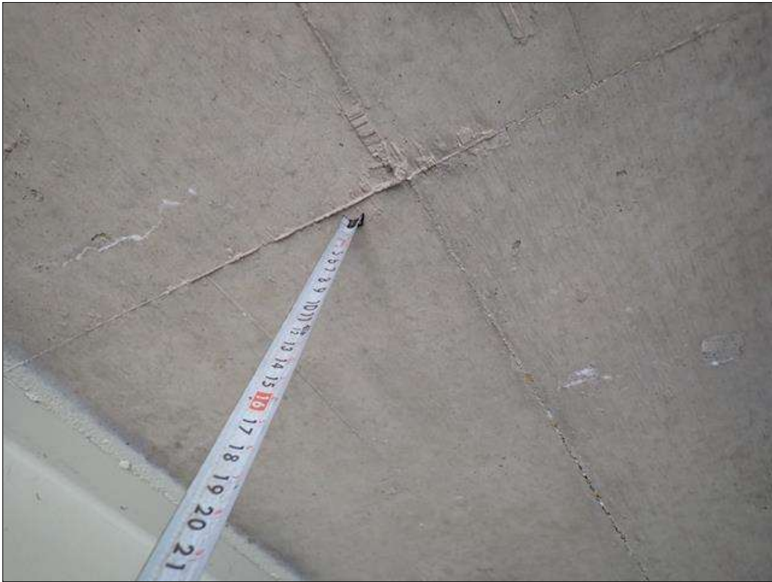
Span 4 Deck: BOTTOM OF DECK HAS MAP CRACKING UP TO 1/64 INCH WITH EFFLORESCENCE IN ALL BAYS.
