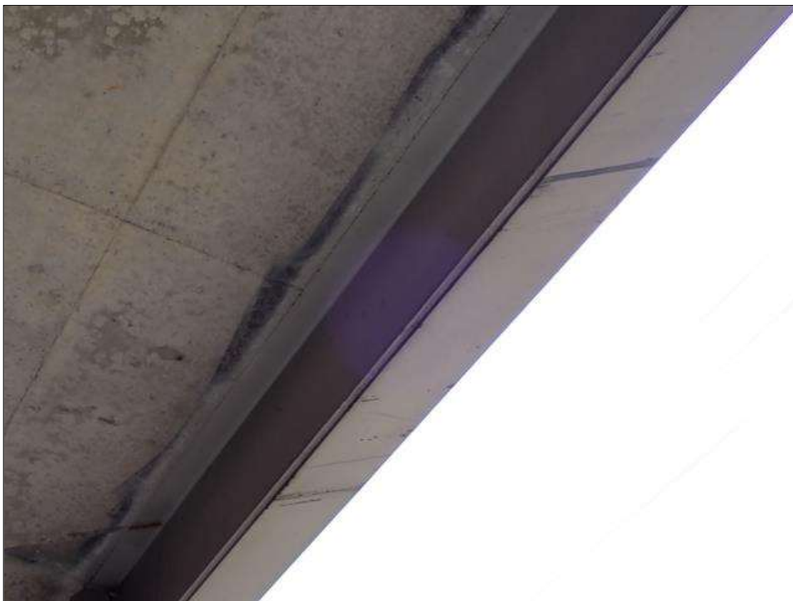
Span 3 Beam 1 - Protective System: over right travel lane, impact scrapes
