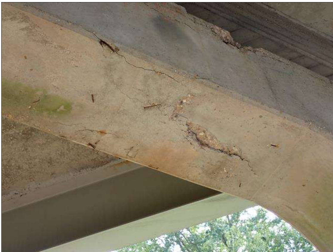
Bent 1 Cap 1: underside of cap, between columns 1 and 3, spalls/delaminations (up to 12 foot x full width x 1 inch deep) with cracks (up to 1/8 inch)
