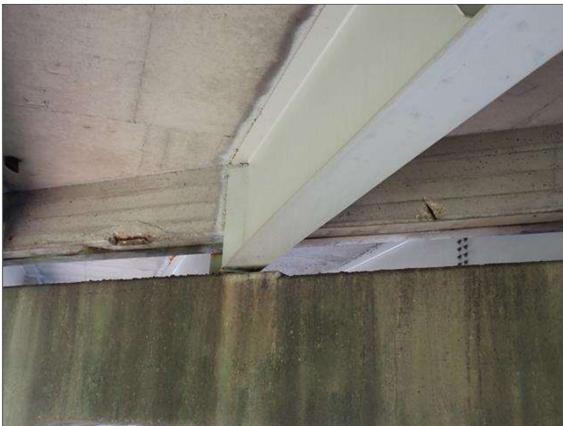
Span 4 Beam 4: UP TO 1 FOOT X 6 INCH X 4 INCH SPALL WITH EXPOSED REINFORCING BAYS 3 AND 4 IN BENT 3 DIAPHRAGM.
