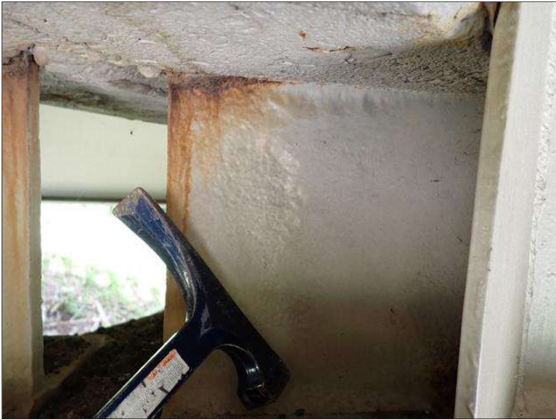
Span 3 Beam 3: at bent 3, pitting with corrosion reactivating: web (up to 1/8 inch deep x 10 inch x 6 inch)
